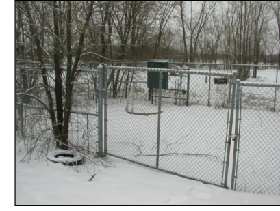
SEWER LIFT STATION ON SUBJECT PROPERTY
