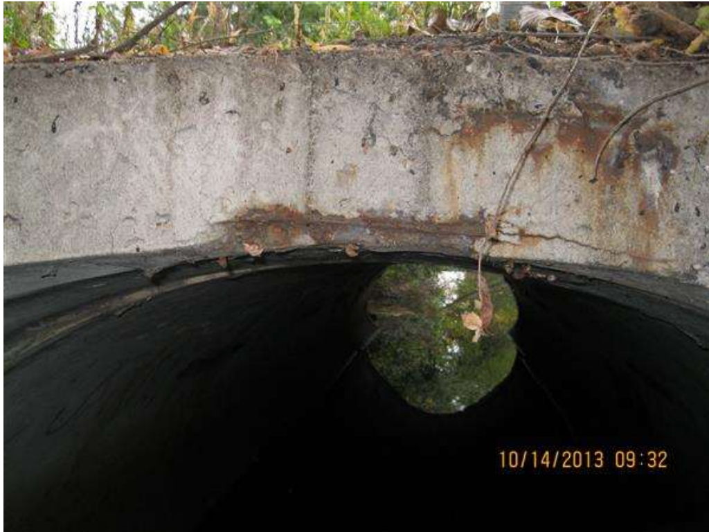
Photo 4 - spall on west end
