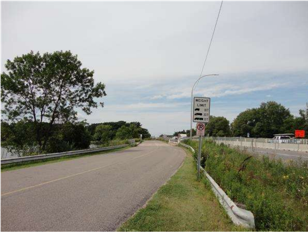
Photo 9 - east load sign 2016
