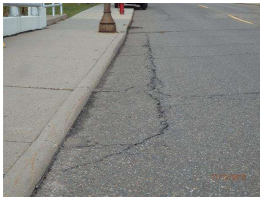
26. longitudinal cracking n-w end of bridge.JPG
