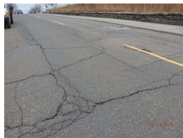
32. north end approach panel cracking and settlement.JPG
