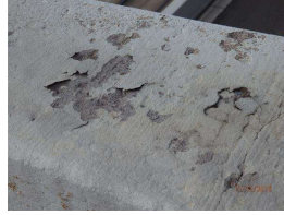
42. top of bridge rail wall - paint peeling typical.JPG
