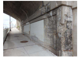
30. north abutment severe spalling -delam.JPG
