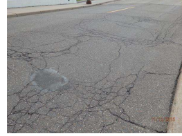
44. various cracking of overlay s-w end.JPG
