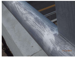
28. metal railing n-w corner paint loss typical.JPG
