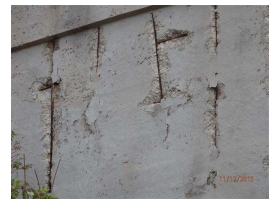
35. north west wing wall severe spalling exposed rebar.JPG
