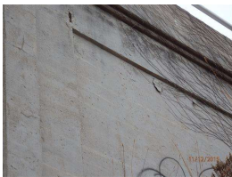
31. north east wing wall - minor spalls.JPG
