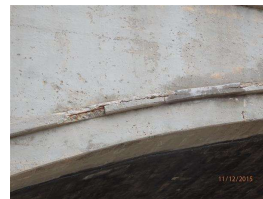
34. north west corner arch barrel delam spalling above west bound traffic removals needed.JPG
