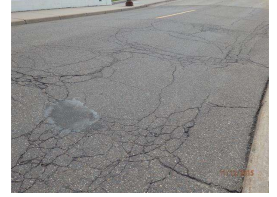
45. various cracking of overlay s-w end (2).JPG
