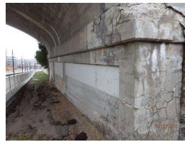
38. south abutment - scalling - spalls - delams.JPG
