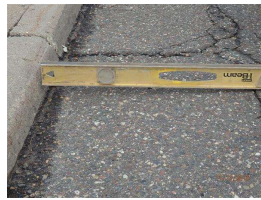
37. settlement at gutter line n-w corner of bridge deck.JPG
