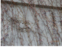
41. south west wing wall - spalls delam.JPG
