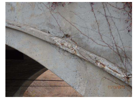
40. south west corner of arch barrel - spalling and exposed rebar.JPG
