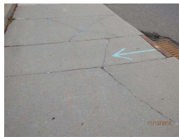
33. north end approach sidewalk cracking.JPG
