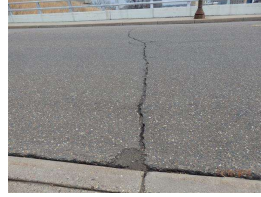
43. transverse cracking mid span west side of bridge.JPG
