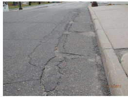
27. longitudinal cracking s-w end of bridge.JPG
