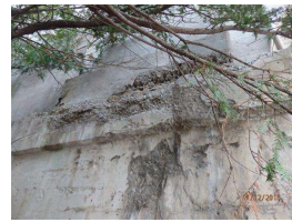
39. south east wing wall - severe spalls delam.JPG
