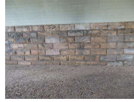
9. N abutment failed mortar joints.JPG
