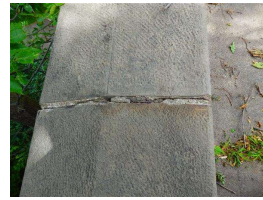
14. stone parapet cape failed mortar joints.JPG
