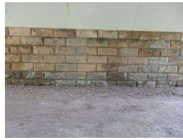
12. S abutment failed mortar joints.JPG
