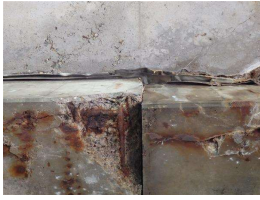
11. Offset of N abut at center looking straight up.JPG
