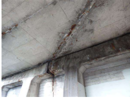
6. Delam at S abut.JPG
