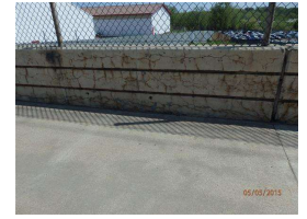
10. bridge rail map cracked.JPG
