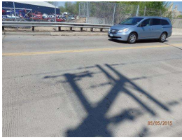
6. approach S.side - cracks.JPG
