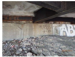
3. abut. South - spalls and delams..JPG
