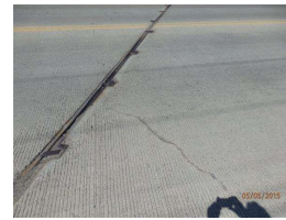
4. approach cracking - N.side.JPG
