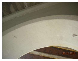
2. 6-17-11 concrete cap cracks.JPG
