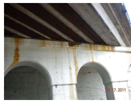
3. 6-17-11 concrete cap spall.JPG
