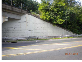
6. 6-17-11 concrete S.wing cracks.JPG
