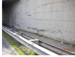
7. 6-17-11 concrete S.wing spalls.JPG
