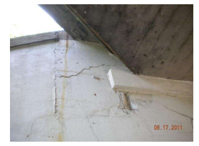
5. 6-17-11 concrete NW.abut cracks.JPG
