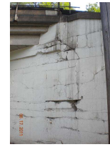
4. 6-17-11 concrete NE.abut cracks.JPG
