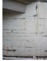
8. 6-17-11 concrete SW.abut cracks.JPG
