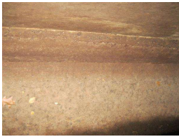
11. spall on south end west culvert.JPG
