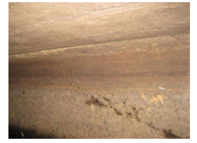
10. spall on south end east culvert.JPG
