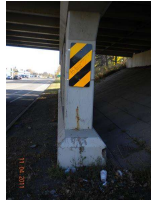
8. column S.side damage_1.jpg
