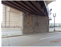
23. north pier wall facing south map cracking and spalls on pier cap.JPG
