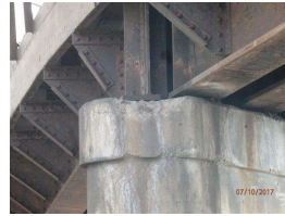
24. north pier wall large spalls exposed rebar.JPG
