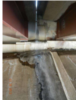
12. CL joint leaking_01.jpg
