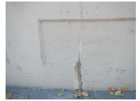
15. parapet rail cracking.jpg
