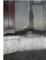
14. CL joint leaking_03.jpg
