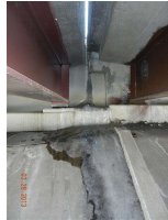
13. CL joint leaking_02.jpg
