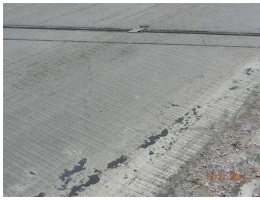
16. approach W.side cracks_2.jpg
