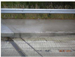
51. Maryland 6599 W. approach_cracks_3.jpg
