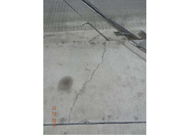
9. approach E.side cracks_1.jpg
