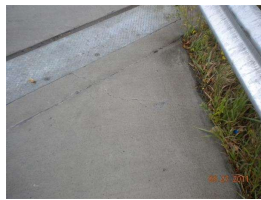
52. Maryland 6599 W. approach_cracks_4.jpg
