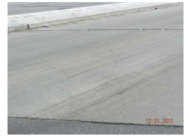
15. approach W.side cracks_1.jpg
