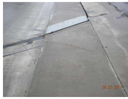
42. Maryland 6599 E. approach_cracks_4.jpg
