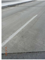
12. approach E.side cracks_5.jpg
