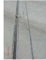
14. approach E.side cracks_7.jpg
