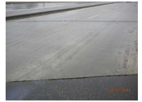
50. Maryland 6599 W. approach_cracks_1.jpg
