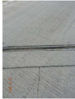
17. approach W.side cracks_5.jpg
