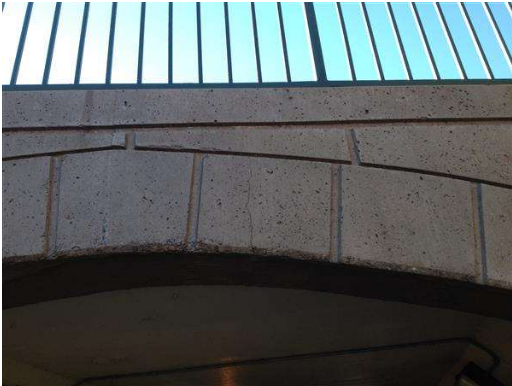
Photo 6 - Crack on west portion of north headwall Looking South
