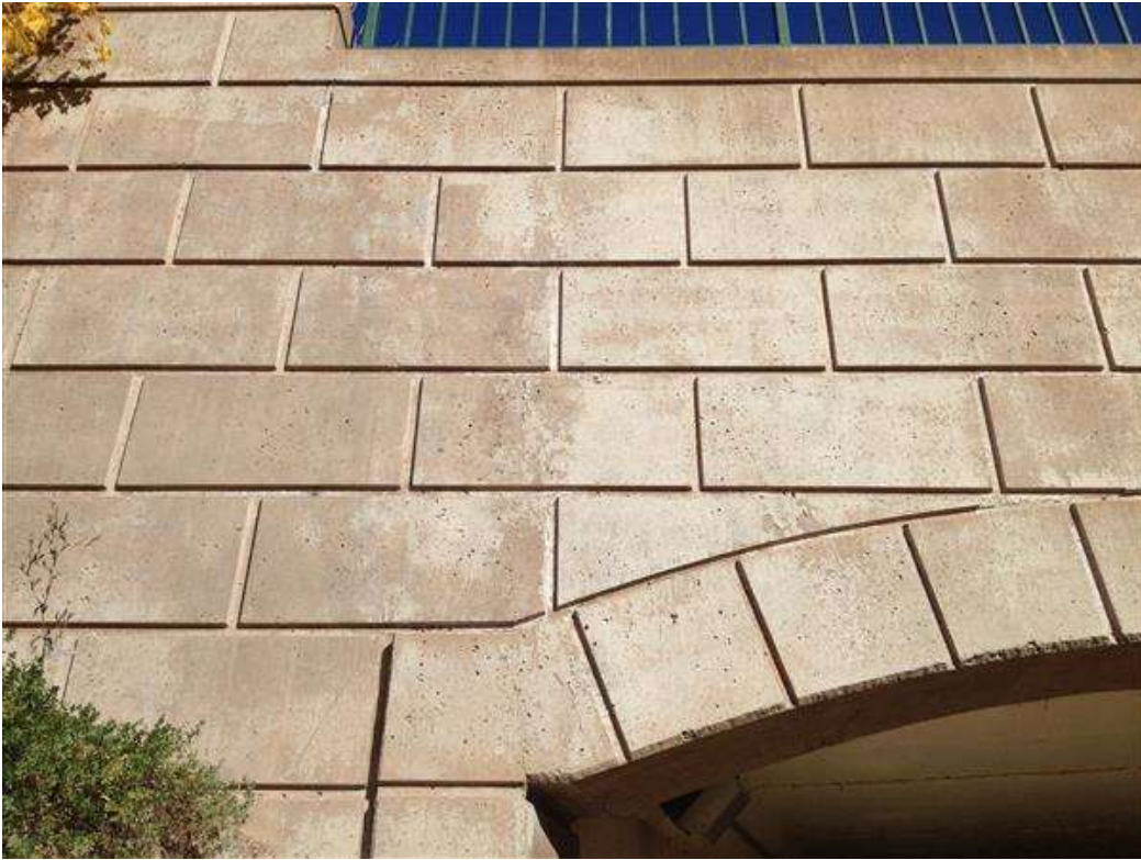
Photo 7 - Hairline crack in west corner of south headwall Looking North
