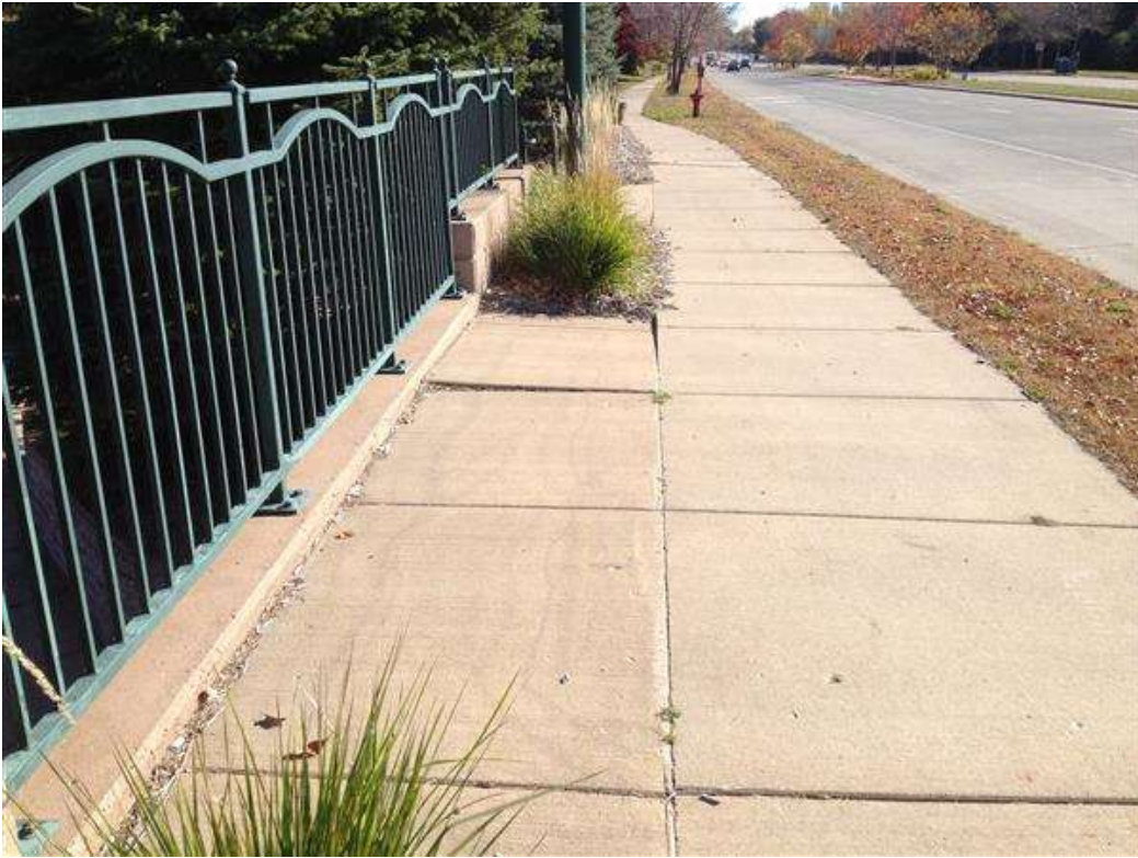
Photo 9 - Tipped panel in north sidewalk Looking East
