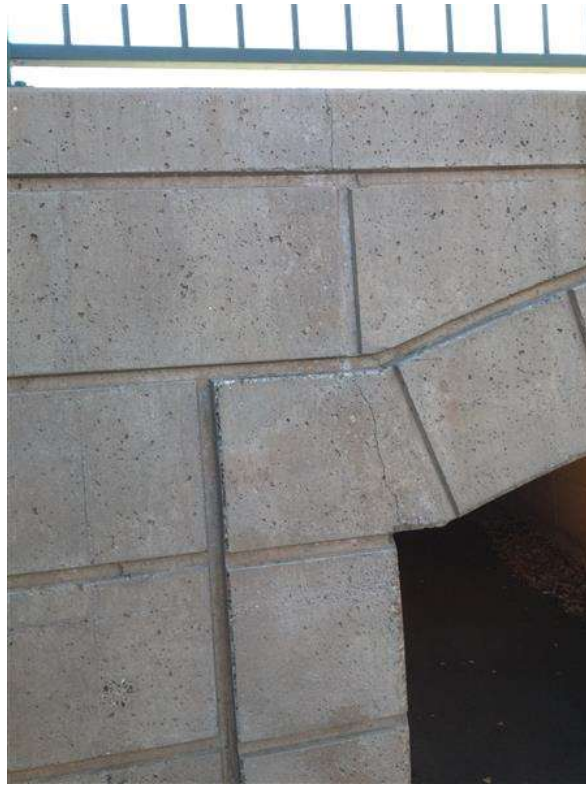
Photo 5 - Crack in east corner of north headwall Looking South
