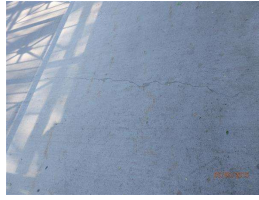
13. transverse cracking of walks.JPG
