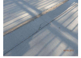
10. approach spall - S.side.JPG
