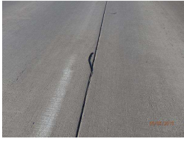
11. joint filler adhesion failure_1.JPG
