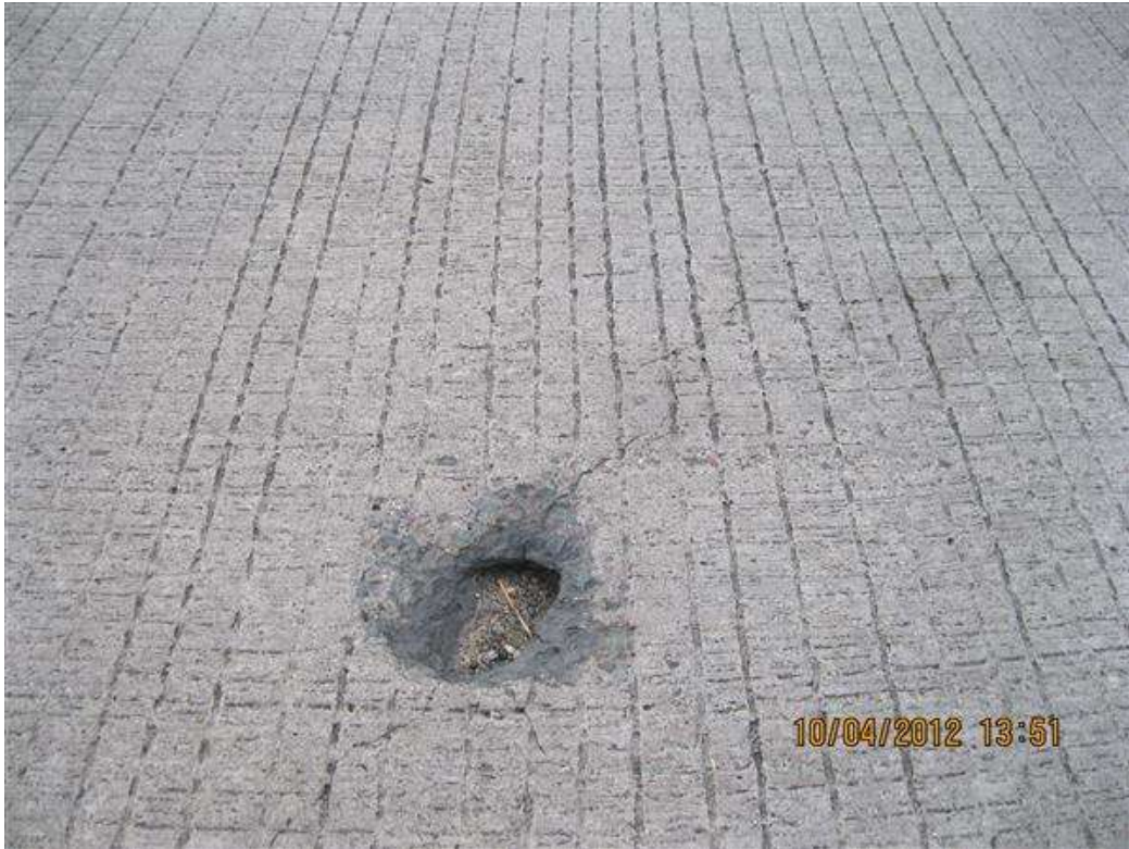
Photo 11 - Overlay South side Pier #1 WB
