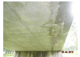
35. underdeck distress E.side_2.JPG
