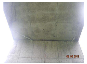
40. underdeck distress E.side_7.JPG
