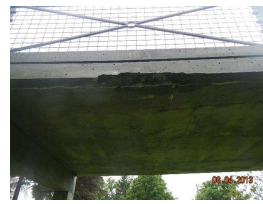
39. underdeck distress E.side_6.JPG
