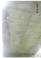
37. underdeck distress E.side_4.JPG
