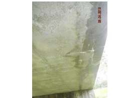
34. underdeck distress E.side_1.JPG
