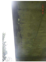
38. underdeck distress E.side_5.JPG
