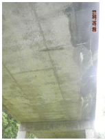
36. underdeck distress E.side_3.JPG
