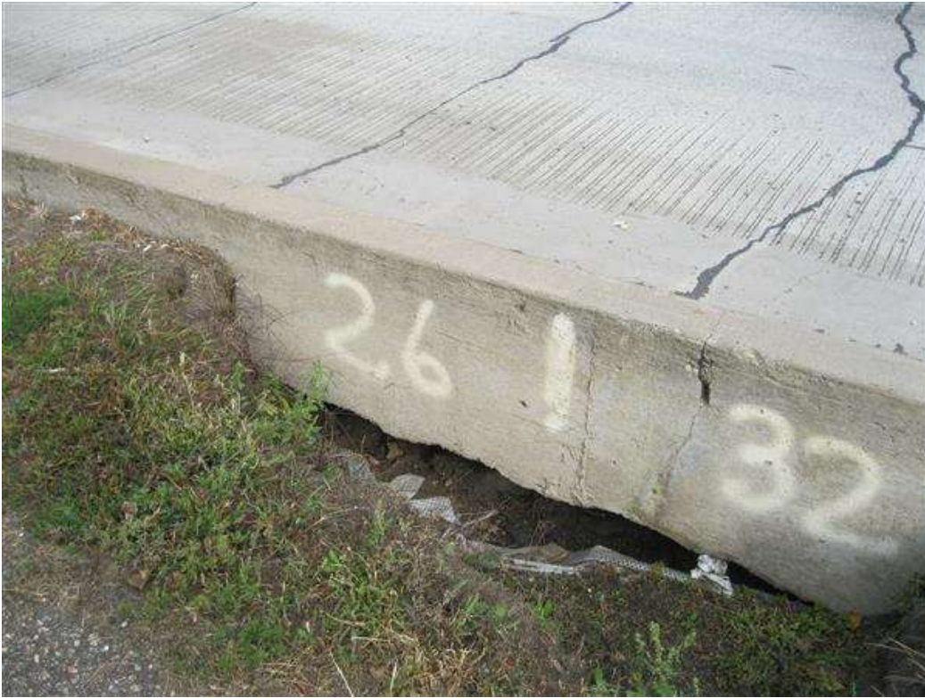
Photo 5 - curb south side-2.JPG
