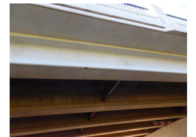
30. 031 E facia girder minor collision damage from traveling W bound on Bush..JPG
