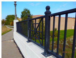
26. 025 NE corner paint failure on railing..JPG
