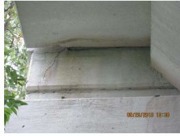
2. Crack in SW Parapet.JPG
