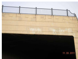
33. Headwall S.end cracks_1.jpg
