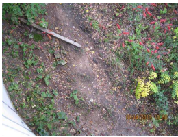
1. erosion @ NW wing wall.JPG
