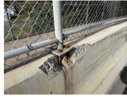
13. West rail spall.JPG
