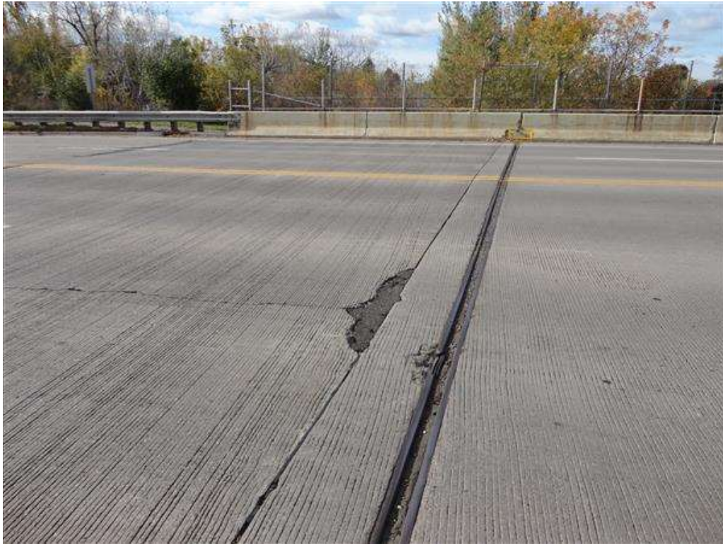
Photo 14 - South approach spall
