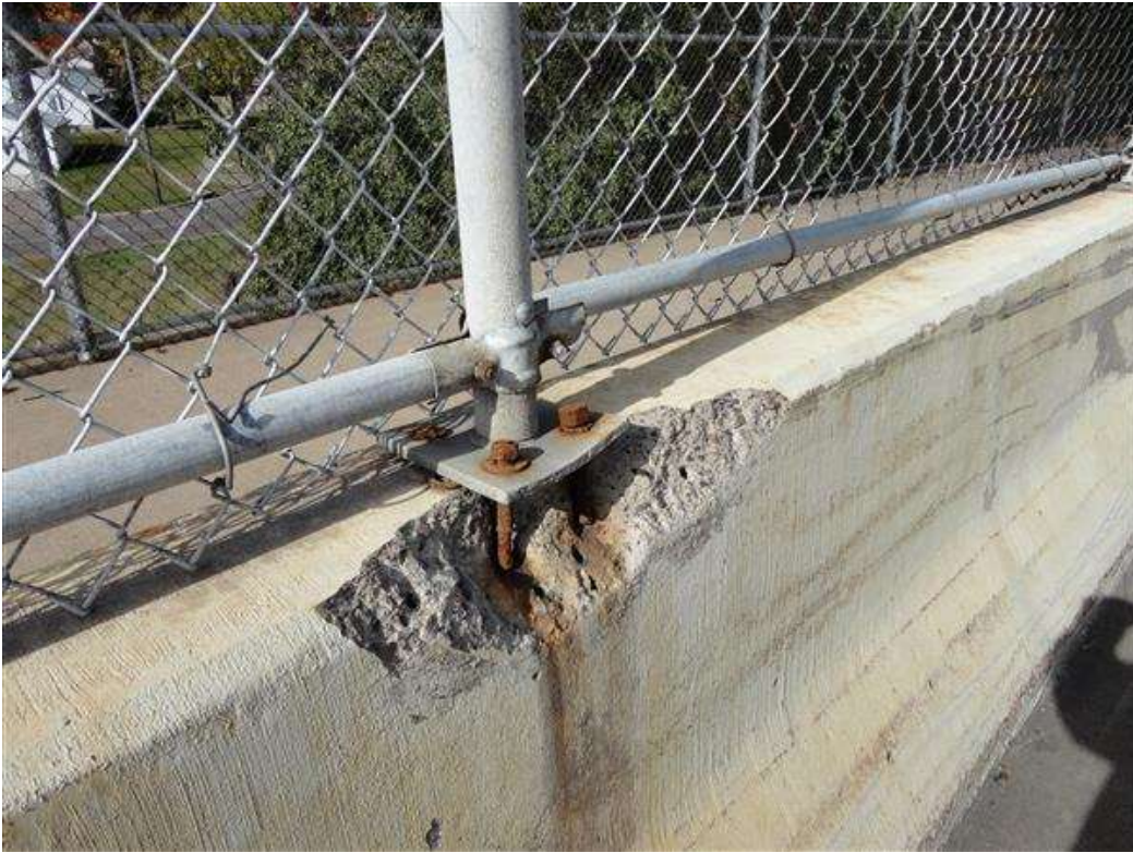
Photo 17 - West rail spall.
