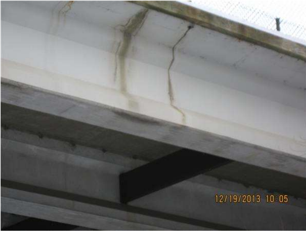
Photo 1 - crack in beam NE corner
