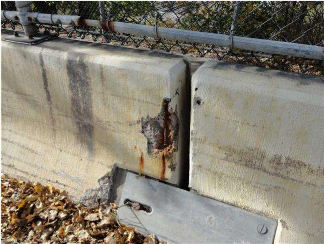
Photo 15 - Spall on east rail
