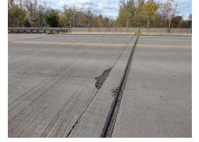
10. South approach spall.JPG
