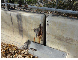
11. Spall on east rail .JPG
