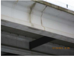
1. crack in beam NE corner.JPG
