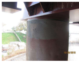
3. 003 Pier 2 north Column 1.5 If Crack.jpg
