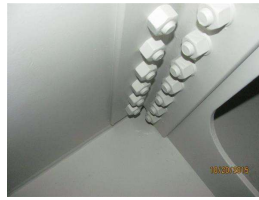
12. 023 Pier 1 Paint Puddled at Beam 5.jpg
