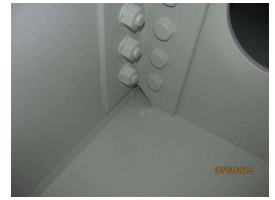
25. 010 Pier 2 Paint Pooled at Beam 6.jpg
