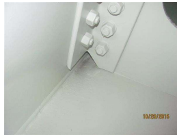
13. 026 Pier 1 Paint Puddled at Beam 7.jpg
