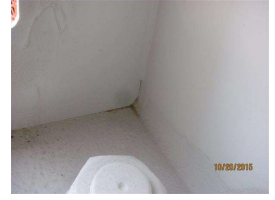
10. 018 Minor Corrosion in the End Diaphragm at the North End.jpg
