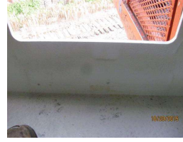
9. 017 Minor Corrosion in the End Diaphragm at the North End.jpg
