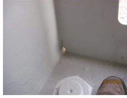
8. 016 Minor Corrosion in the End Diaphragm at the North End.jpg
