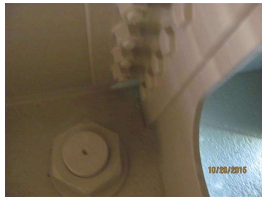
11. 027 Pier 1 Cracked Paint at Beam 1.jpg
