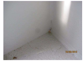
20. 015 Minor Corrosion in the End Diaphragm Corners at the South End.jpg
