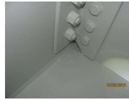
24. 011 Pier 2 Paint Pooled at Beam 5.jpg
