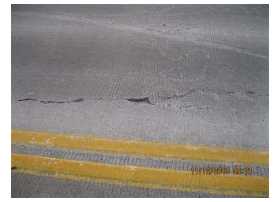
5. spall on deck.JPG
