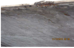
6. spall under deck east side near north pier.JPG
