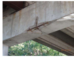
4. 4th pier from east abut spalling.JPG
