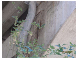
2. 3rd pier from east abut spalling.JPG
