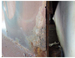
12. south abut. beam end flaking rust.JPG
