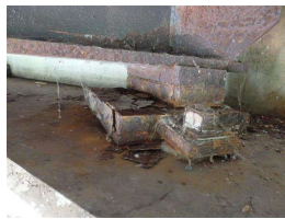
18. south abut. expansion bearing heavy rust heavy flaking.JPG
