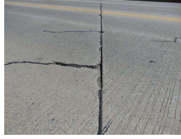
8. liquid poured joint sections missing.JPG
