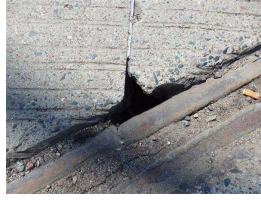
7. hole in deck south abut repairs needed.JPG
