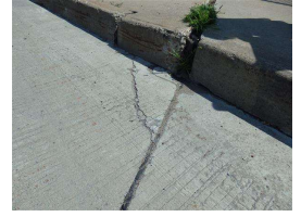
10. north east approach small delamination.JPG
