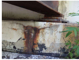
22. southwest abut. 2lf delam.JPG
