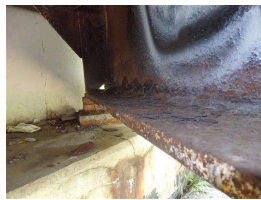
17. south abut. end of beam flaking rust.JPG
