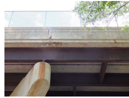
24. west side back side parapet wall spalls and cracking.JPG
