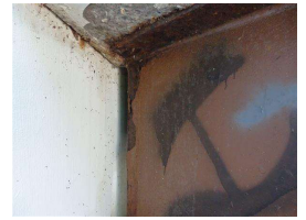
15. south abut. east end flaking rust.JPG
