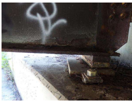
16. south abut. end of beam flaking rust (2).JPG
