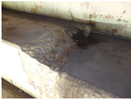
21. south abut. large spall.JPG
