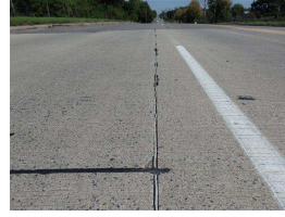
9. north abut. adhesion failure.JPG
