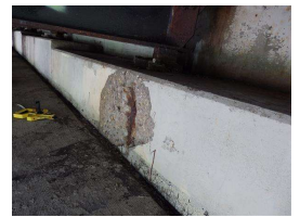
20. south abut. large spall (2).JPG
