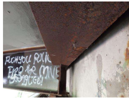
13. south abut. bottom of diaphragm flaking rust.JPG
