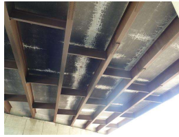
23. underside of deck map cracking leaching efflor..JPG
