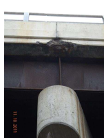
28. underdeck spall at cold_joint_2.jpg
