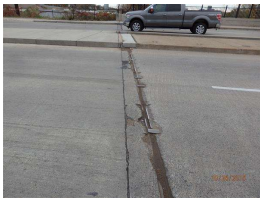
16. 028 E approach unsound patches in paving block..JPG
