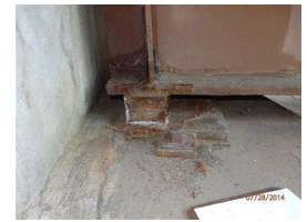
5. bearing corrosion 034.JPG
