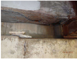
6. 019 W end concrete diaphragm delams and spalls..JPG
