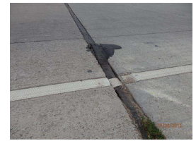
15. 027 E approach liquid poured joint failure..JPG
