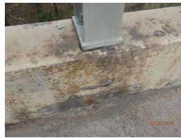
17. 029 E end, S side of parapet, spalls and delams..JPG
