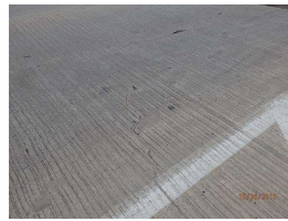
13. 025 W approach sealant failure..JPG
