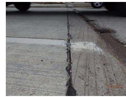
14. 026 E approach liquid poured joint failure..JPG
