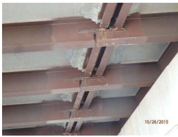
11. 023 W pier hinge bearings, corrosion and paint failure..JPG
