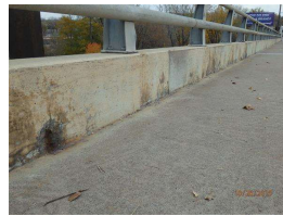
18. 030 W end, S side of parapet, spalls and delams..JPG
