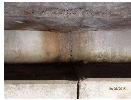
3. 018 Vertical cracking W abut at back wall..JPG
