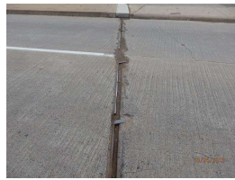
12. 024 W strip seal armor extrusion failure..JPG
