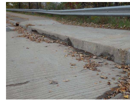
19. 031 NW corner approach sidewalk undercutting..JPG
