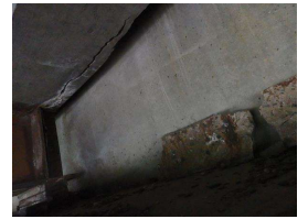
30. Spall with exposed rebar center bay S end.JPG
