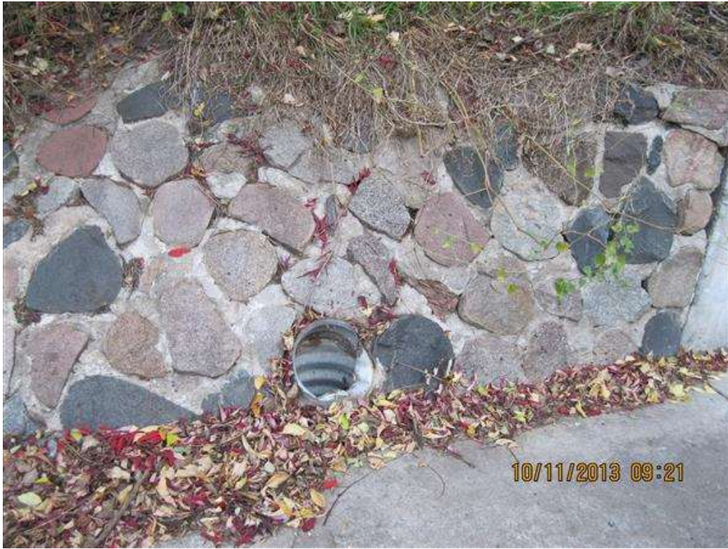
Photo 1 - drain on nw cor
