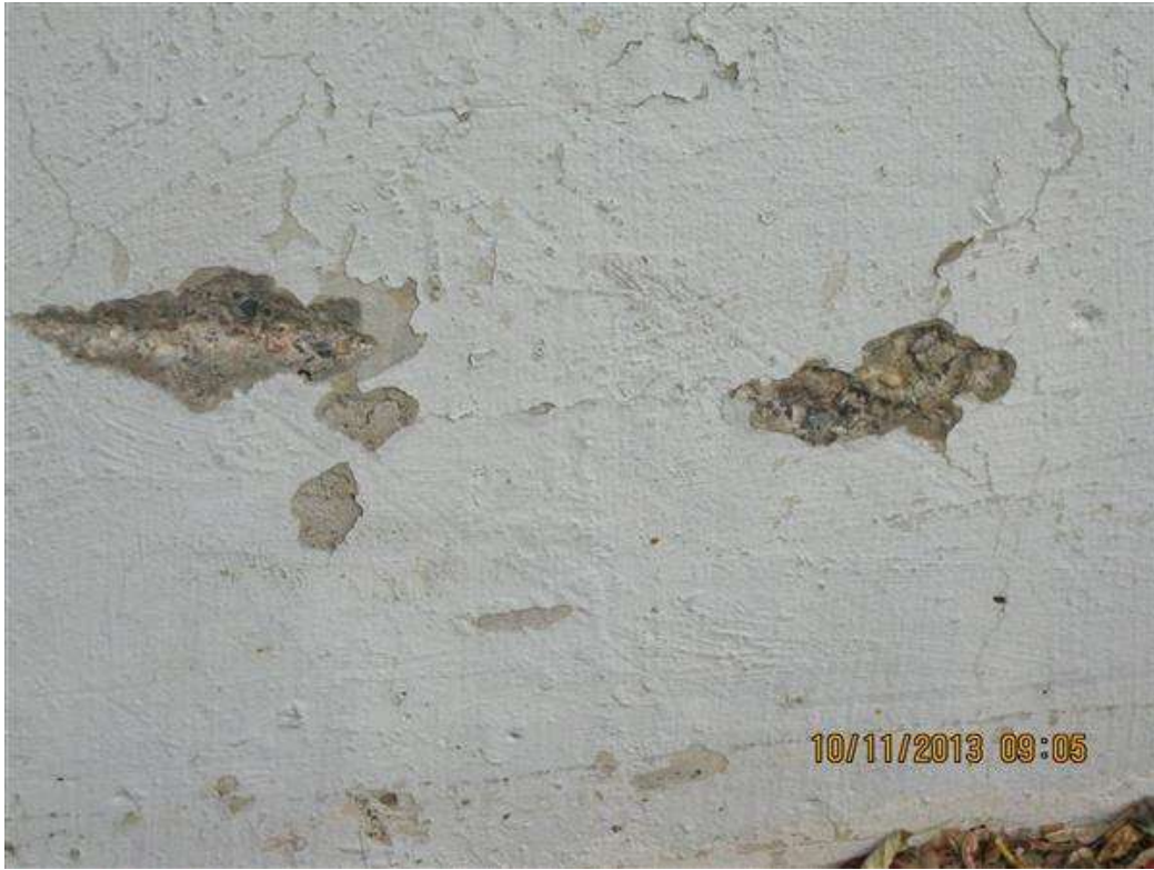
Photo 9 - spalls on NE cor
