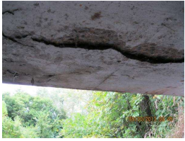
1. Delamination west end north culvert .JPG
