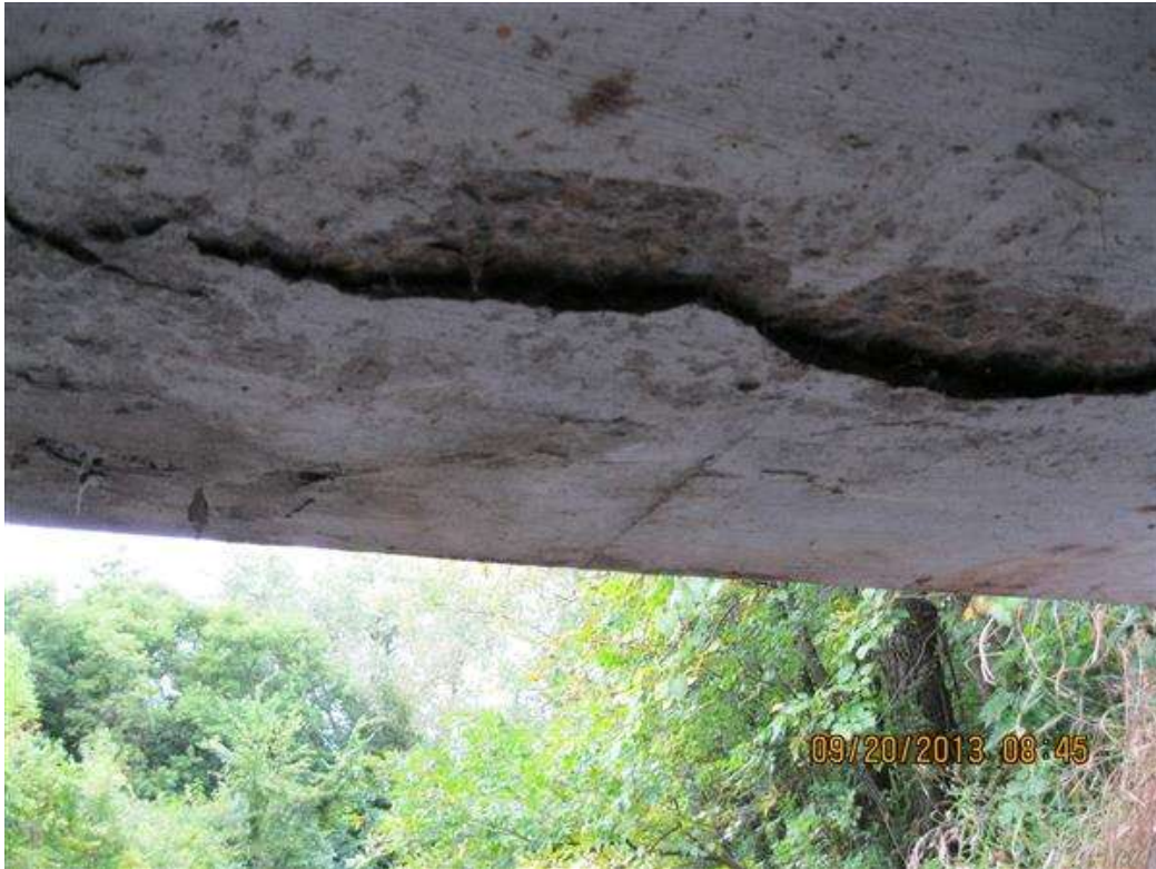
Photo 1 - Delamination west end north culvert 2013
