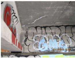
1. crack under bridge.JPG
