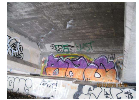
5. more cracks under bridge.JPG
