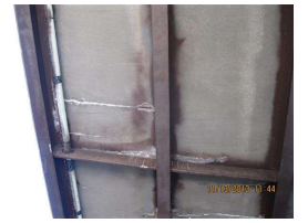
5. spall & crack under deck.JPG
