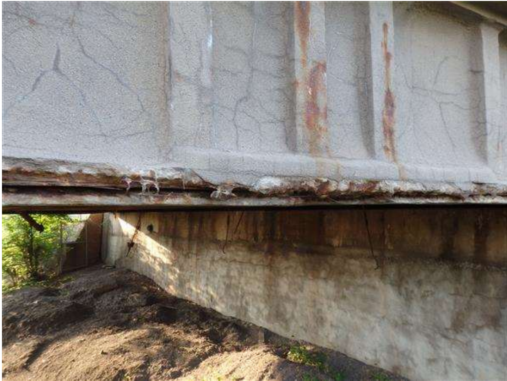
Photo 10 - abut SW fascia b mapcracking
