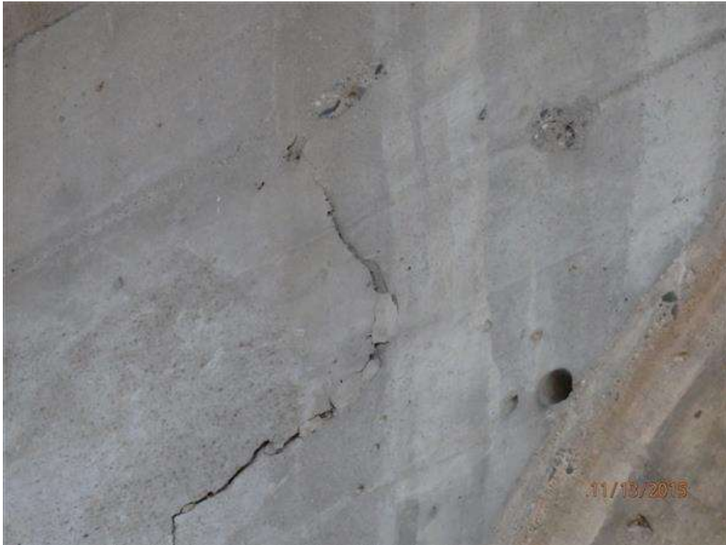
Photo 4 - center column pier 1 - delam south face
