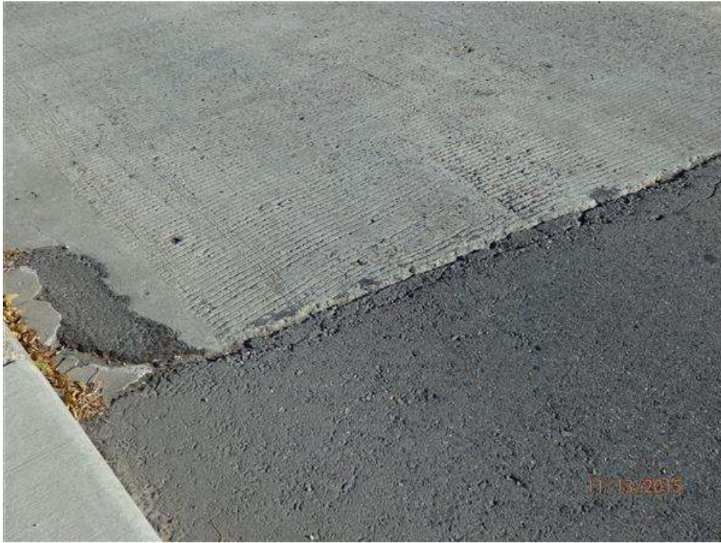
Photo 21 - unsound patch SW approach panel
