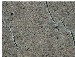
18. unsealed cracks on sidewalk - typical.JPG
