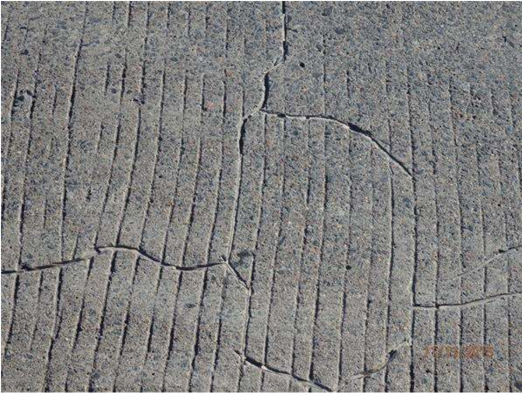
Photo 17 - unsealed cracks on deck - typical
