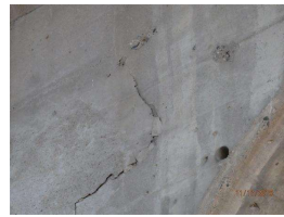
4. center column pier 1 - delam south face.JPG
