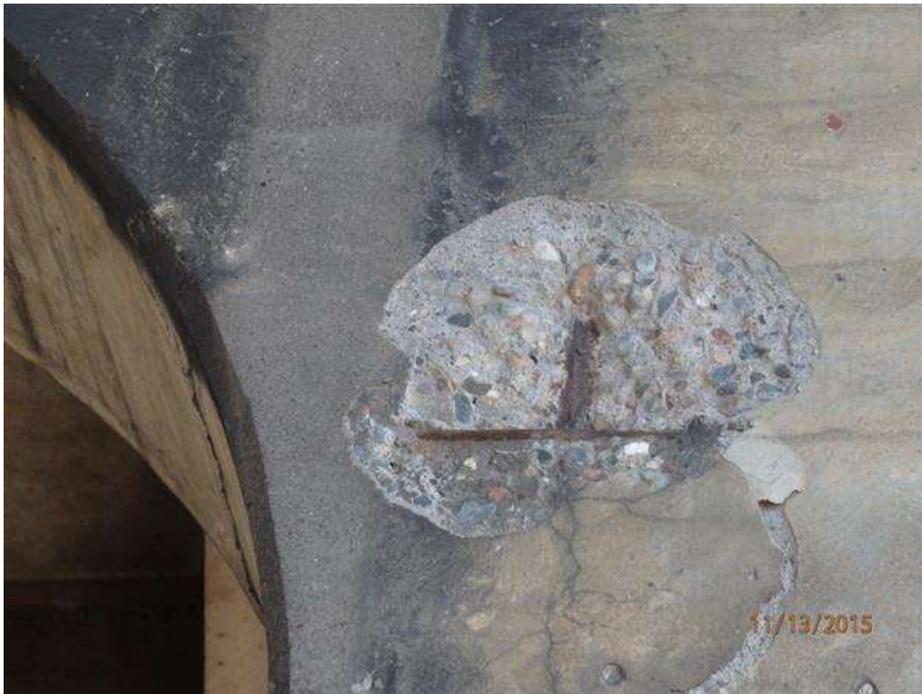
Photo 8 - column spall pier 2 south face
