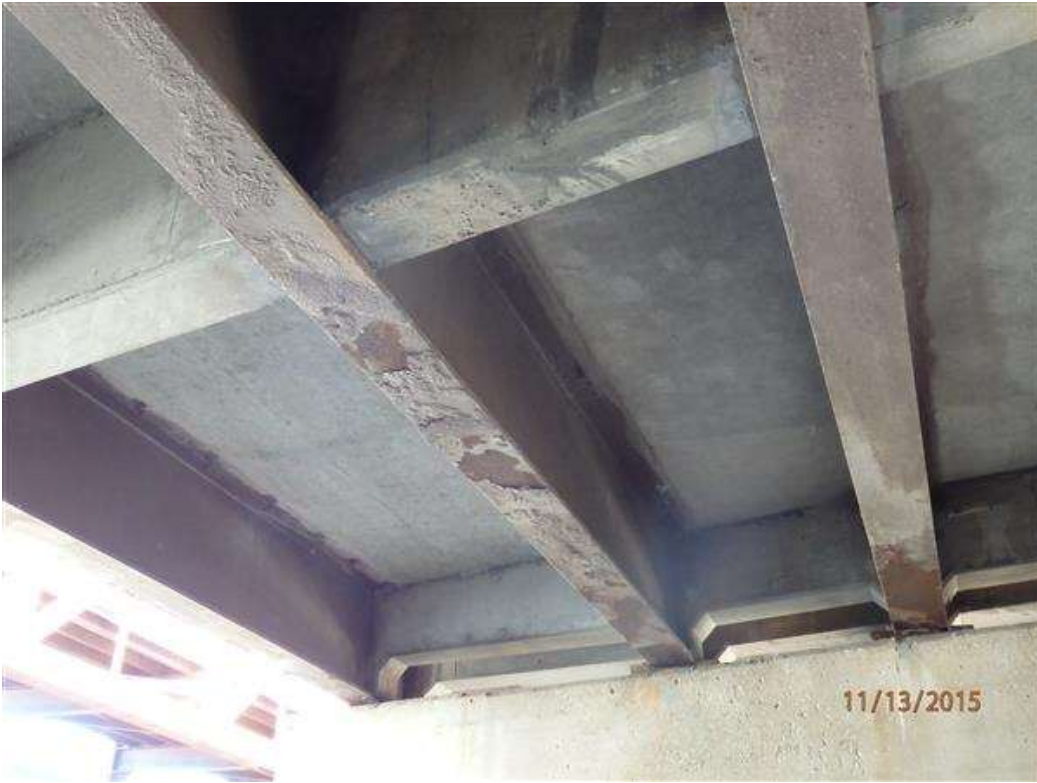
Photo 3 - beam ends pier 4 - rusty
