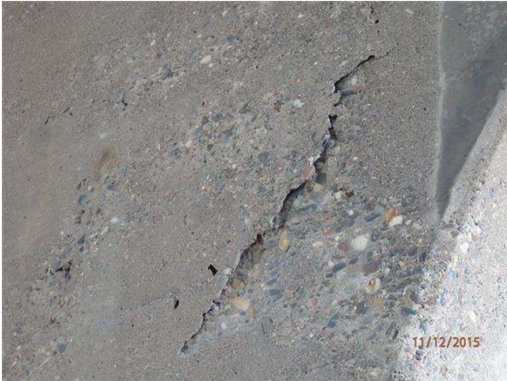
Photo 9 - column spall pier 4 south end
