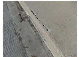
30. Southbound curb at S end.JPG
