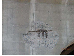
7. column spall pier 1 south face.JPG
