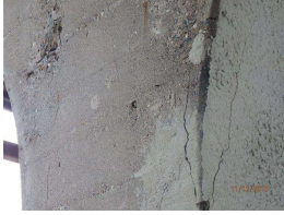
6. column delam - spalls pier 4 south end.JPG
