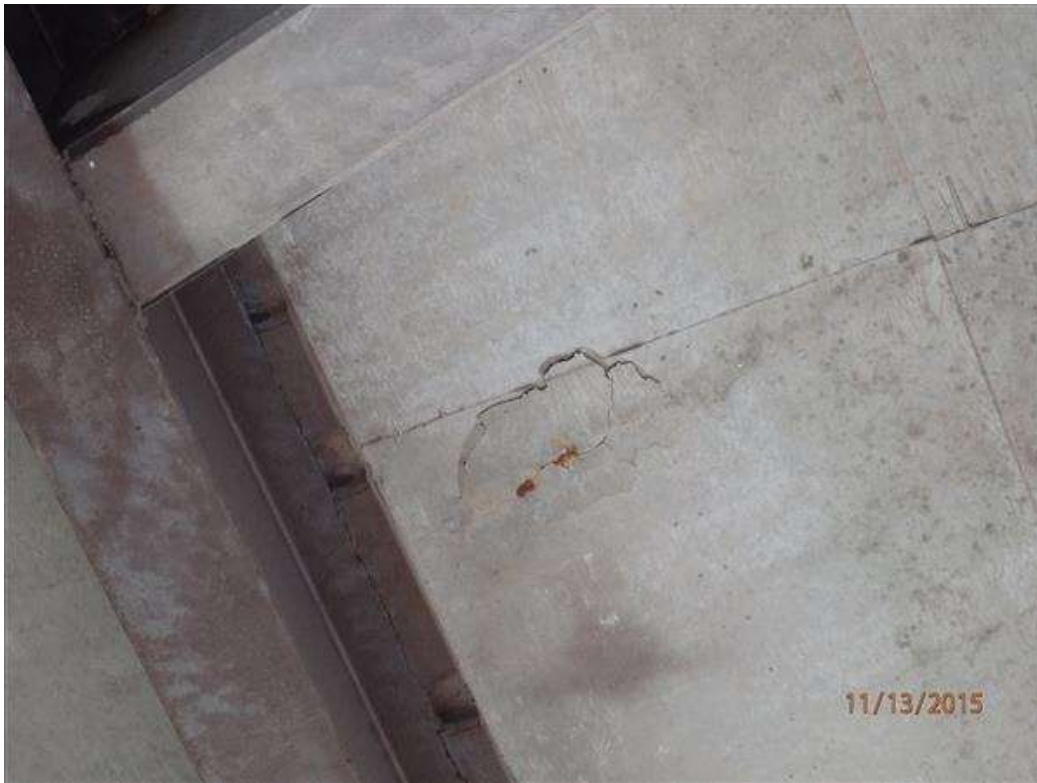
Photo 15 - underside of deck between pier 4 and pier 3 has delam
