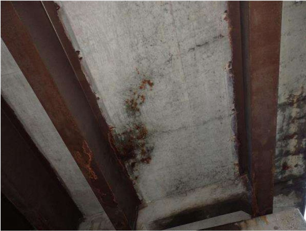
Photo 31 - Staining, E side near S abut
