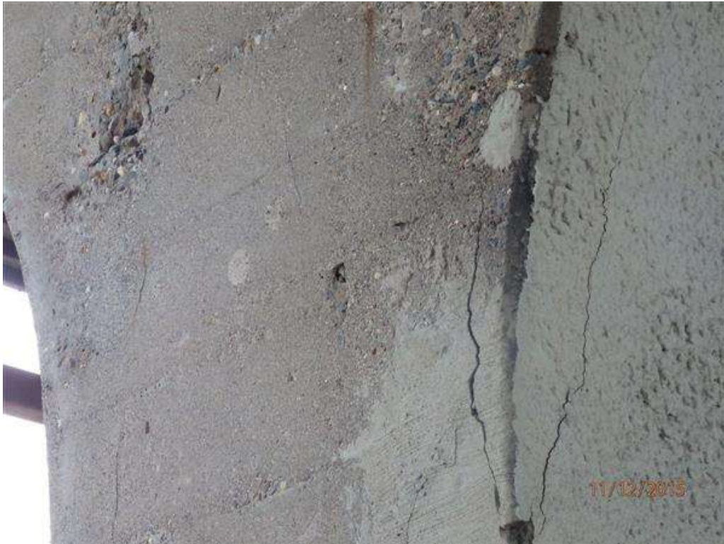
Photo 6 - column delam - spalls pier 4 south end
