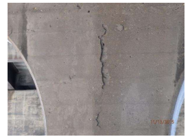
5. center column pier 1 spalls north face.JPG
