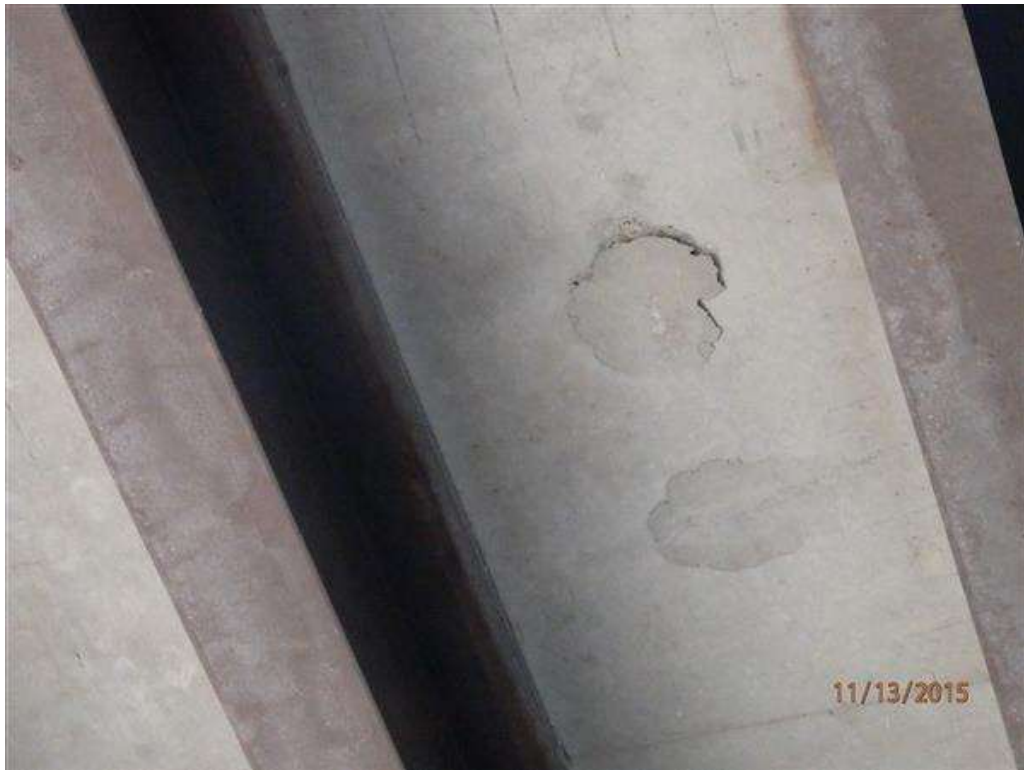
Photo 16 - underside of deck between pier four and pier three has delam
