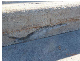
13. longitudinal cracking at curb face east side mid span.JPG
