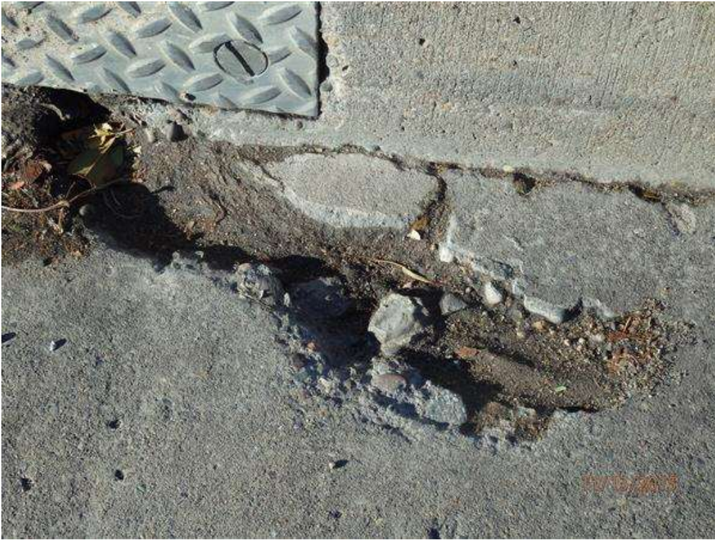
Photo 19 - unsound patch NW approach panel at gutter line
