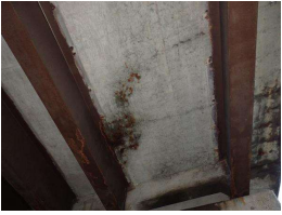
31. Staining, E side near S abut.JPG
