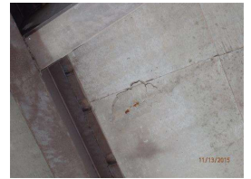
15. underside of deck between pier 4 and pier 3 has delam.JPG
