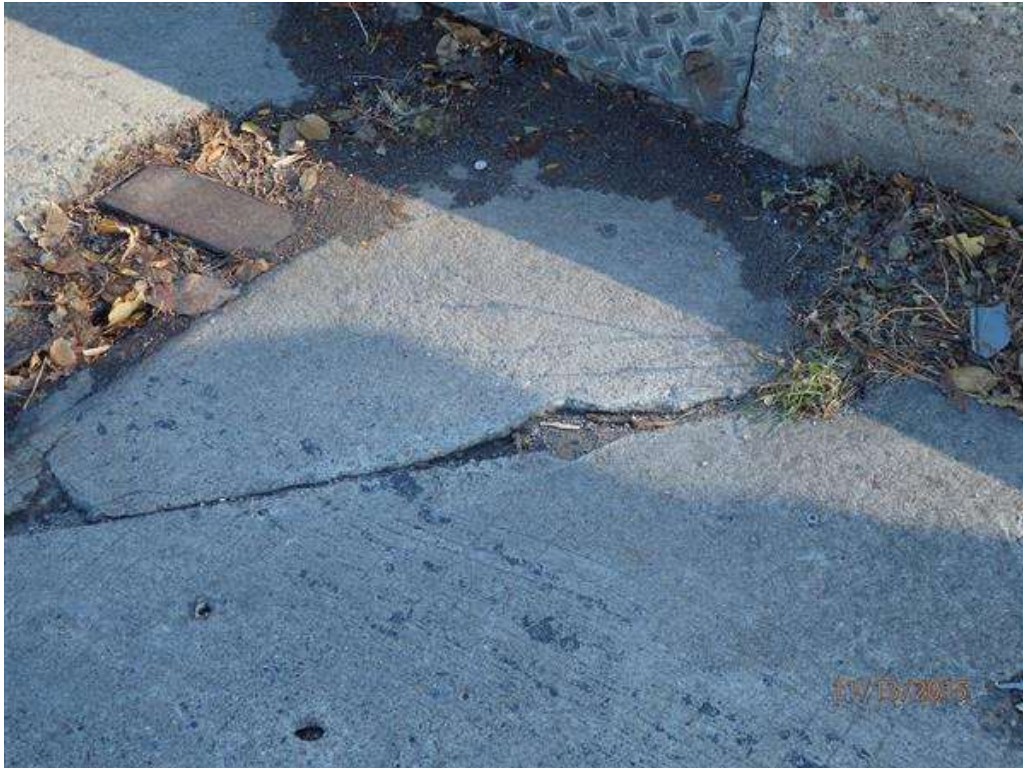
Photo 20 - unsound patch S. approach panel at gutter line
