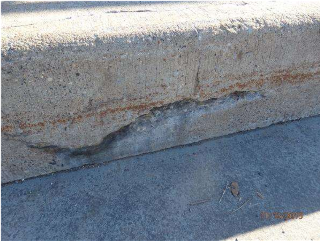
Photo 13 - longitudinal cracking at curb face east side mid span
