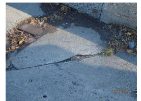
20. unsound patch S approach panel at gutter line.JPG
