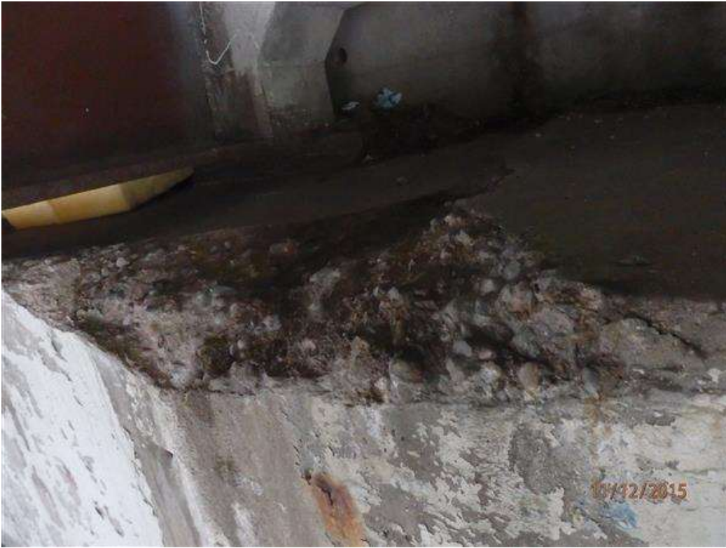
Photo 1 - abut seat SW - spalls - exposed rebar - leakage
