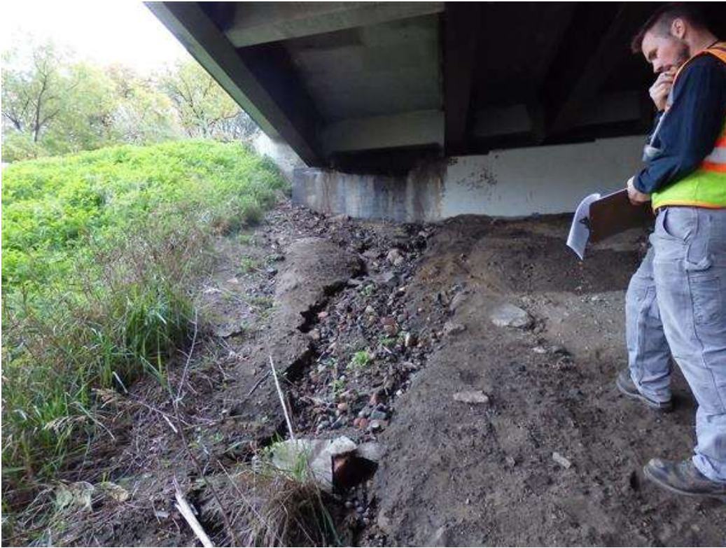
Photo 29 - Slope washout at SE end
