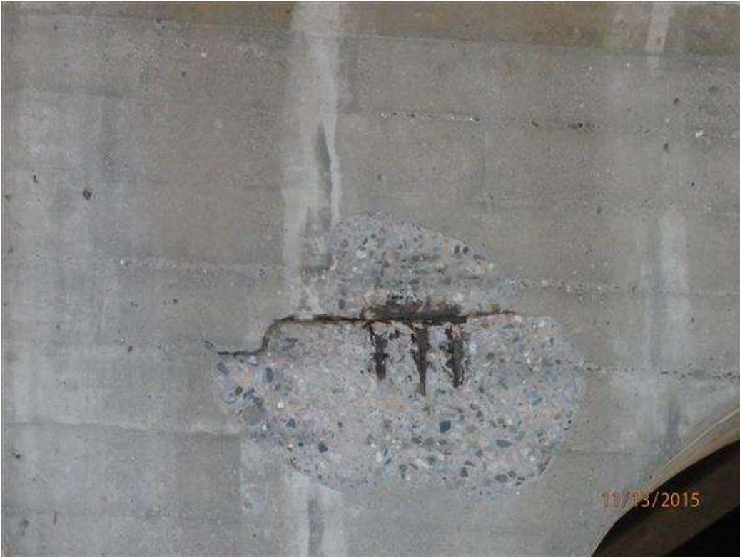
Photo 7 - column spall pier 1 south face
