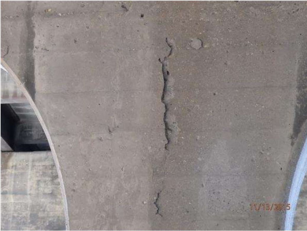
Photo 5 - center column pier 1 spalls north face
