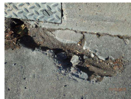
19. unsound patch NW approach panel at gutter line.JPG
