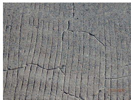
17. unsealed cracks on deck - typical.JPG
