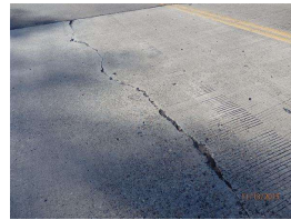
14. longitudinal cracks south approach panel.JPG
