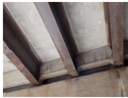
2. beam ends pier 1 - rusty - north face.JPG
