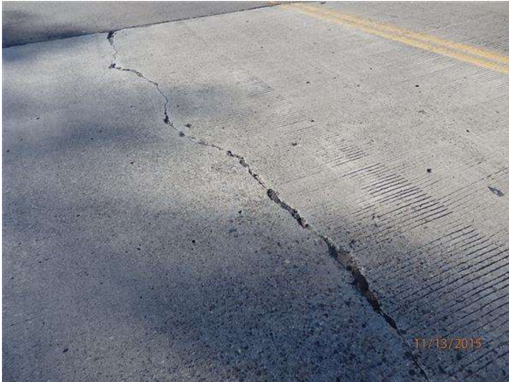
Photo 14 - longitudinal cracks south approach panel
