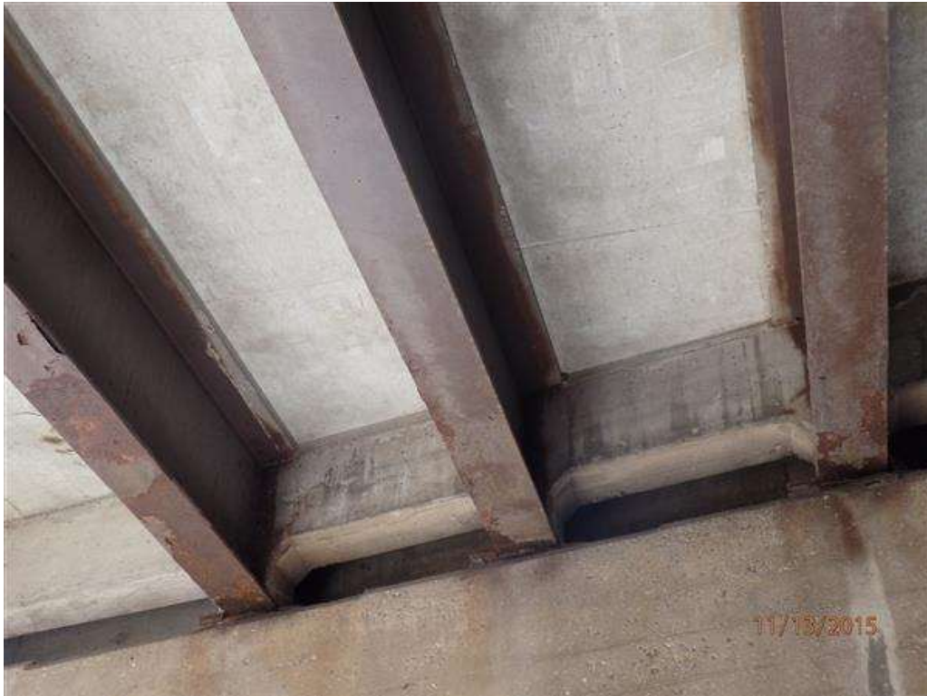
Photo 2 - beam ends pier 1 - rusty - north face
