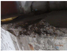
1. abut seat SW - spalls - exposed rebar - leakage.JPG
