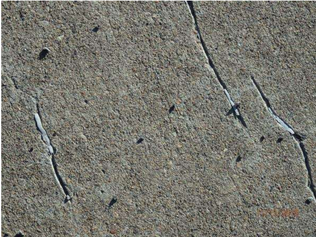
Photo 18 - unsealed cracks on sidewalk - typical
