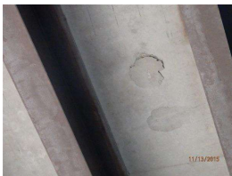
16. underside of deck between pier four and pier three has delam.JPG
