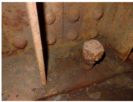
1. anchor bolt corrosion east abut center span.JPG
