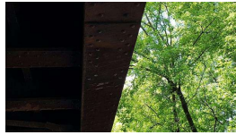
7. N girder sheared rivets.jpg
