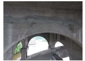
5. 021-spandrel beam cracking Unit 3 btw e-f, ns.jpg
